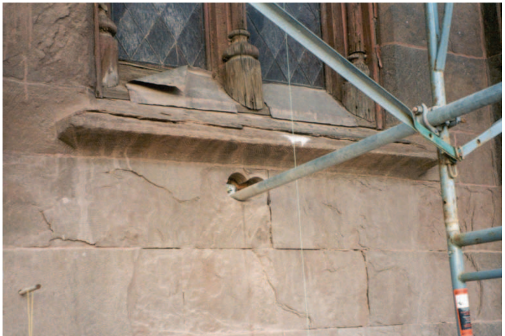
Scaffold stand-off going through the stone veneer attaching to the structure back-up system.
