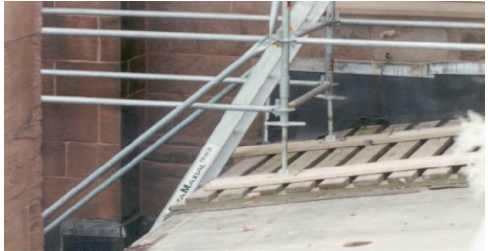
Scaffold tower legs supported directly on roof with cribbing to distribute loads over the roof.
