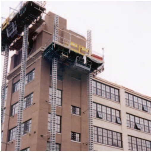
Mobile scaffold towers with tie-ins properly attached to the structure through the brick veneer.
