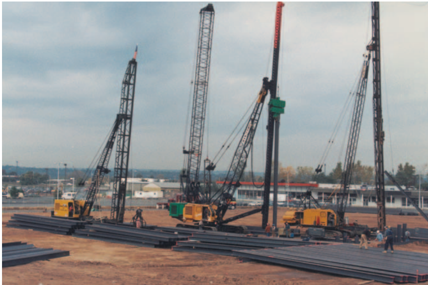
Driving steel H-piles with a vibratory hammer, and seating with an impact hammer.
