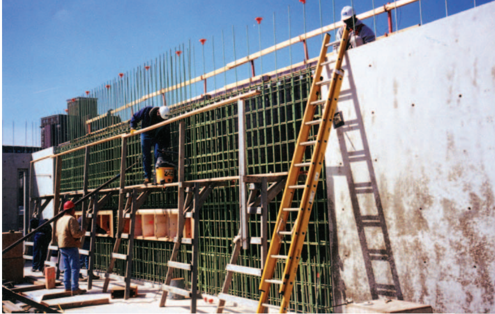
Pictured above: Epoxy-coated reinforcing bars and leak-proof forms at block-outs and construction joints were necessary to achieve a nearly blemish-free concrete
