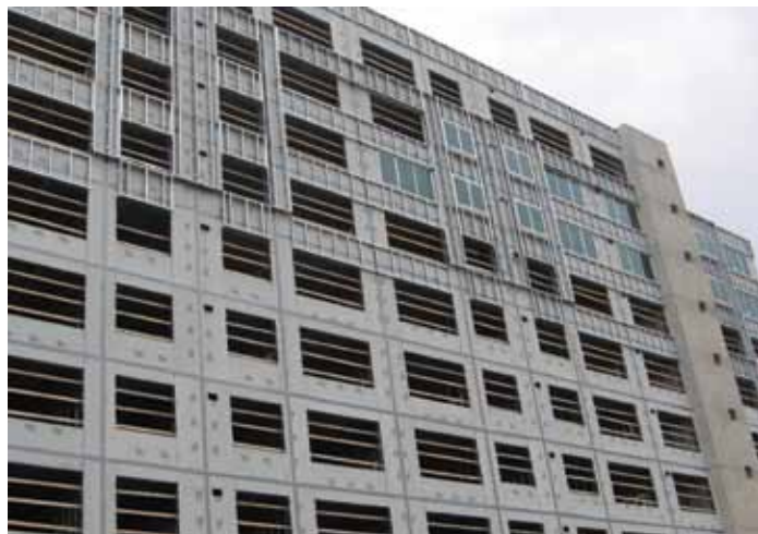
Figure 5. Exterior cold-formed steel framing the primary load-bearing system for the top eight floors.
