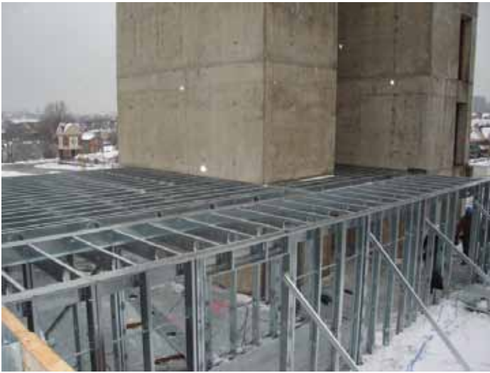
Figure 3. The design features pre-fabricated cold-formed steel joists, rim track and structural blocking.
