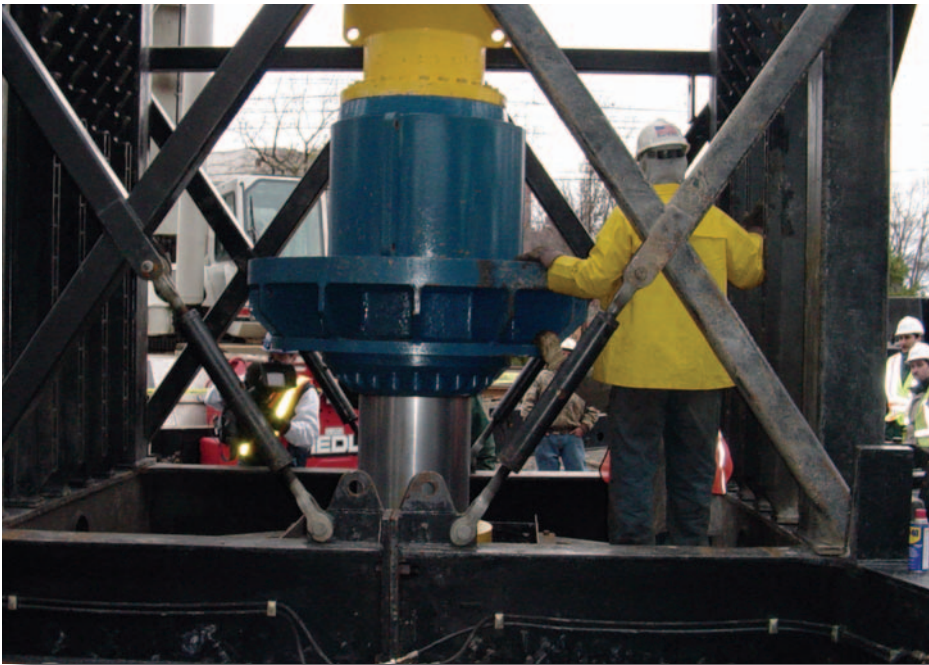
Figure 5: Statnamic Pitson (with load cell and displacement sensor) mounted on top of shaft, Stratford, CT
