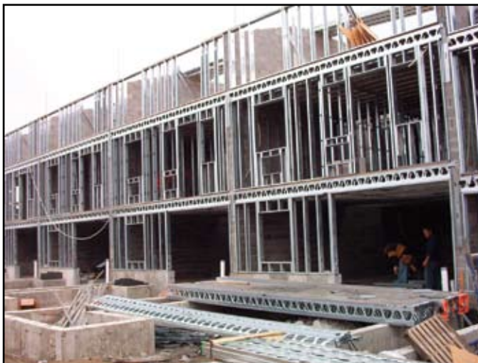
Multi-story load bearing structure using perforated joists. Photo Courtesy of Marino\Ware, Inc.
