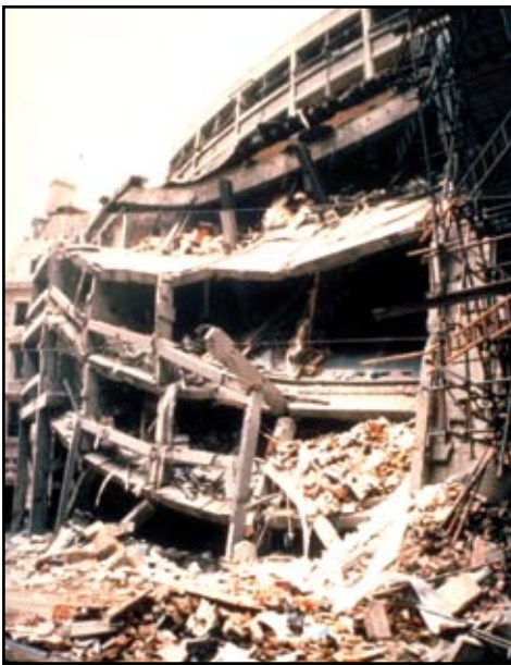
Figure 2: Blast Damage to the Chamber of Shipping Building in St. Mary Axe, London, 1992. ©Arup
