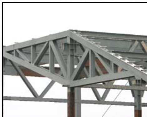
Figure 3: Photo of 75 foot long by 14 foot high typical prefabricated raker truss, which was designed to maximize shop assembly and simplify erection.
