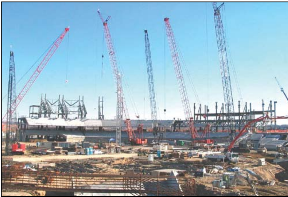
Figure 5: Simultaneous construction activity including earth work, pile installation, cast-in-place concrete forming and placement, steel erection, and precast erection.
