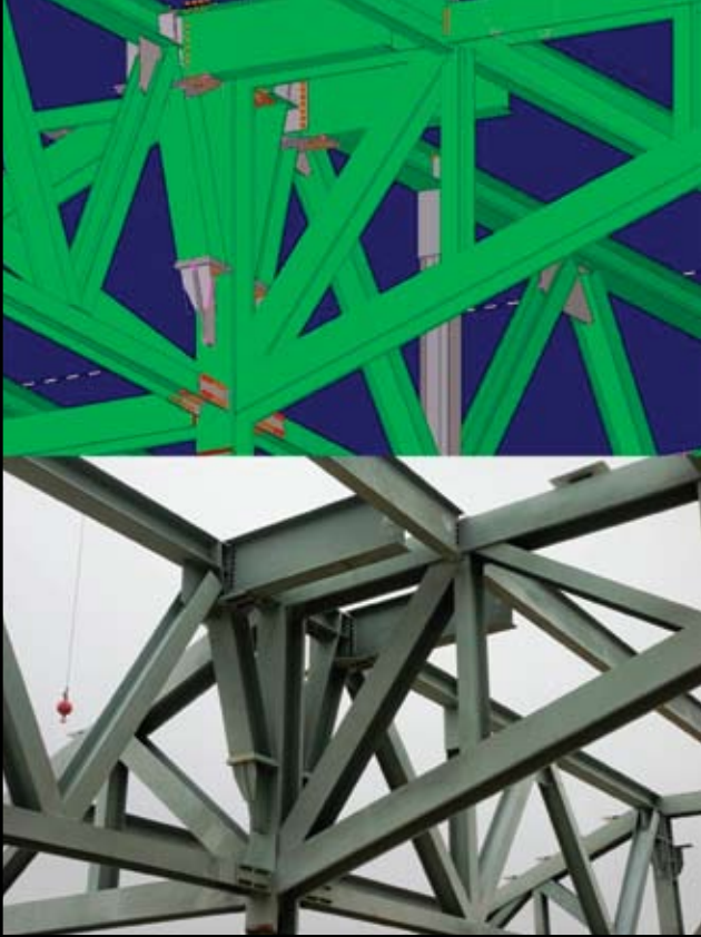
Figure 2: View from the Tekla model (above), Courtesy of Mountain Enterprises. Actual in place steel (below) Courtesy of Thornton Tomasetti
