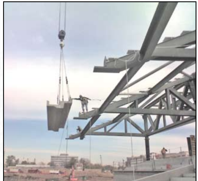
Figure 4: Start of precast seating-tub erection. Staged structural analyses were performed to allow precast erection prior to complete construction of the steel frame.
