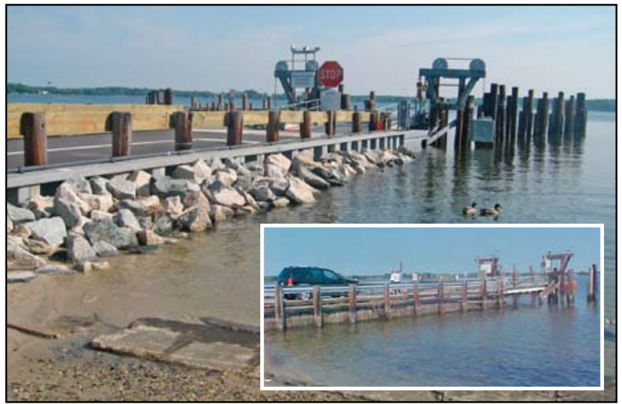
Figure 1: Ramp and approach after reconstruction (May 2006). Inset - Ramp and approach before reconstruction (October 2004)
