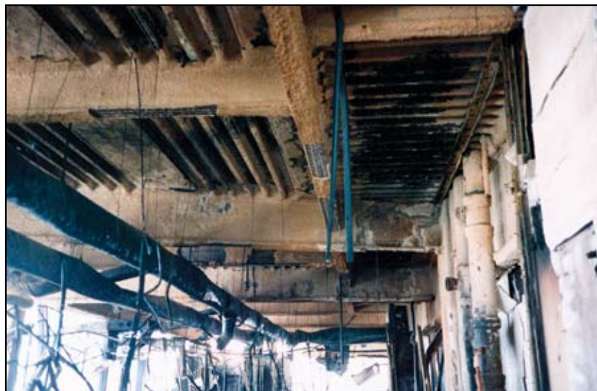
Better Performance: Office Building Fire. Beams Girders and Columns remained intact. Some fireproofing removed from the steel as a result a result of the stream of water from the Fire hoses, but the building survived the fire.
