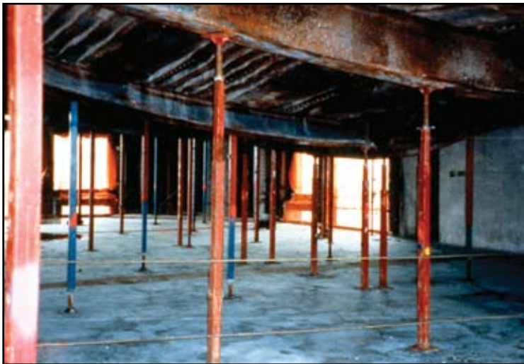
Poor Performance: Office Building Fire. Beams and Girders sagging severely. Result of intense heat over a number of hours.
