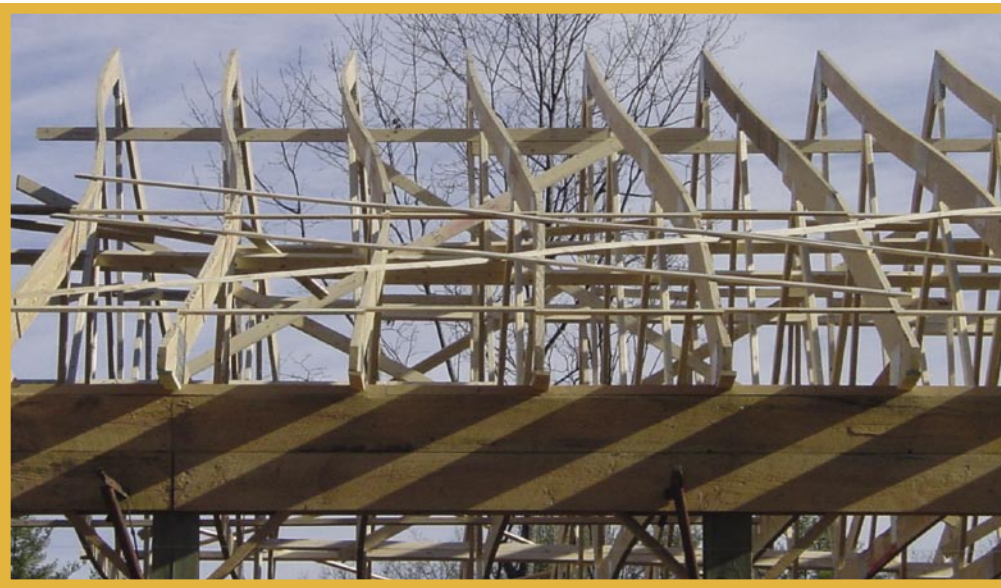
Inadequate Bracing of Trusses
