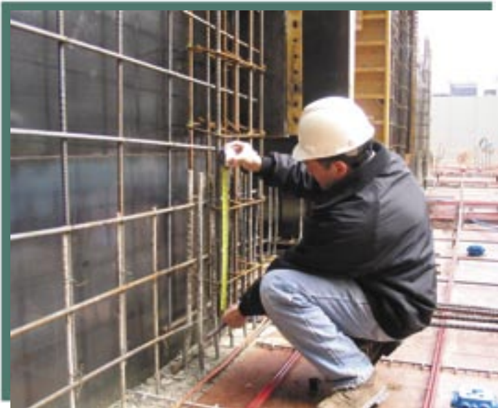
Requirements for location and minimum lengths for splicing of reinforcement must be provided by the engineer
