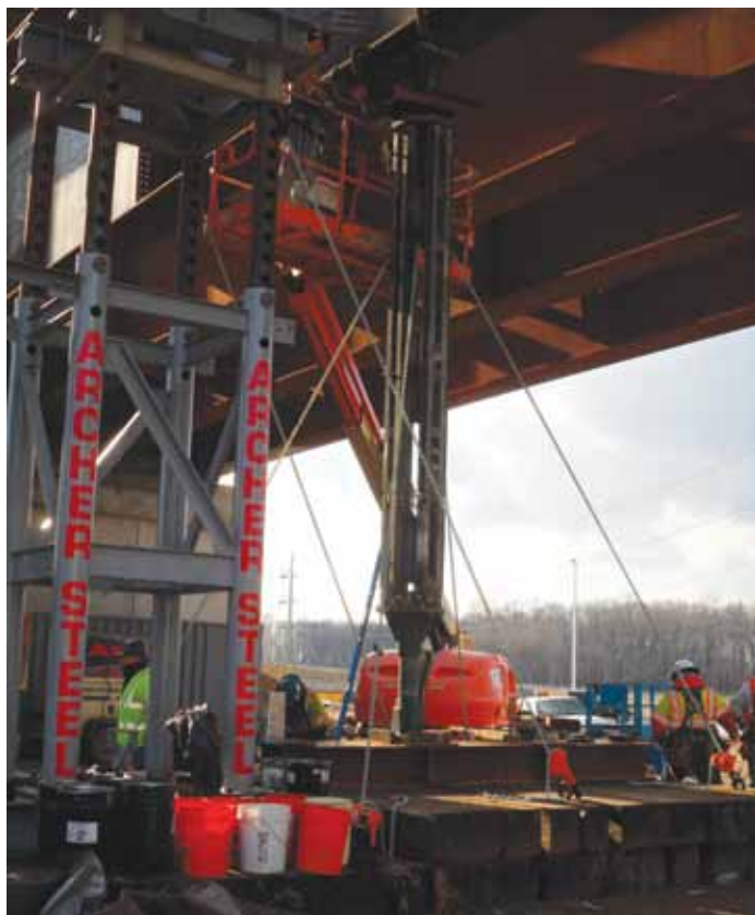
Figure 4. Jack Post A beneath Girder Line 4 and tower for support of Girder Line 5.
