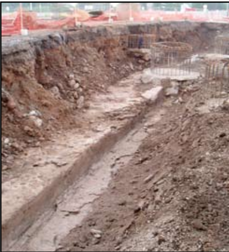
Ledge cut into rock at canal edge. Note drilled pier straddling the edge.
