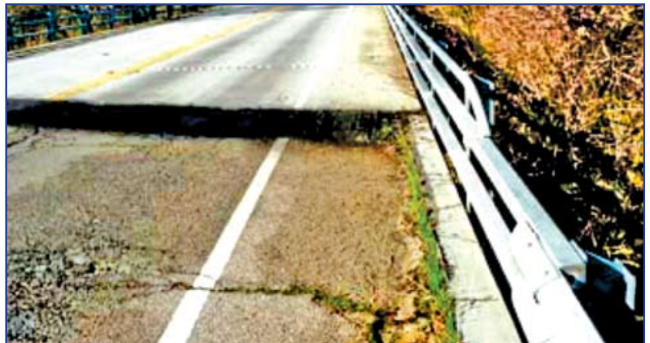
Figure 3: Bridge approach settlement due to liquefaction during the M 6.5 San Simeon earthquake of December 22, 2003. Source: EERI (2004).
