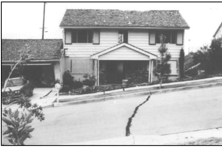
Figure 4: Street and house damaged by several inches of landslide displacement during the M 6.6 1971 San Fernando Earthquake. Displacement is readily visible as street crack in photograph. Source: Applied Technology Council, ATC (1994).
