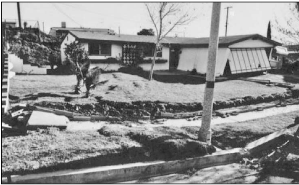
Figure 2: House damaged by surface fault rupture from the M 6.6 1971 San Fernando Earthquake. Source: Applied Technology Council, ATC (1994).
