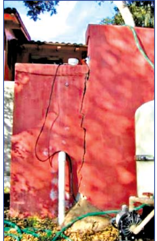
Figure 5: Retaining wall damage from the M 6.5 San Simeon earthquake of December 22, 2003. Granular backfill spilling from new crack in retaining wall.
