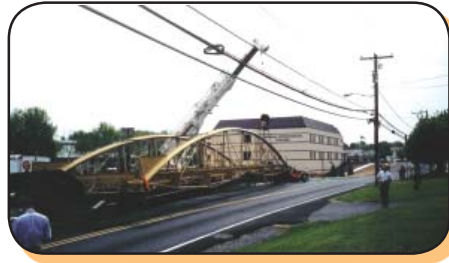
Crane waiting for bridge to be backed into Tech Center parking lot
