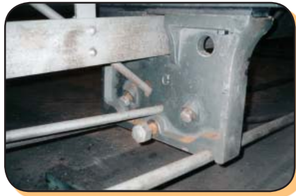
Cast iron strut block and iron sag rod added to brace bottom chord
