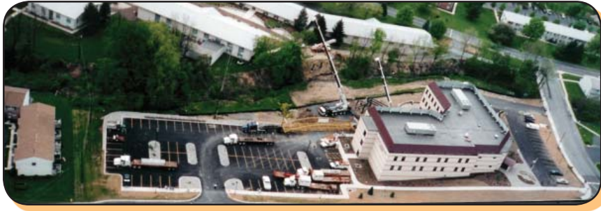
Bridge needed into place adjacent to steam separating residential portion of campus from new Tech Center — cranes are in place
