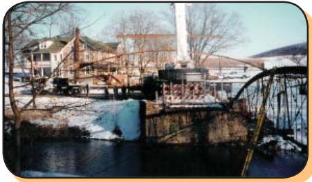
Arch number 1 being lowered onto trailer; arch number 2 being prepared for lifting
