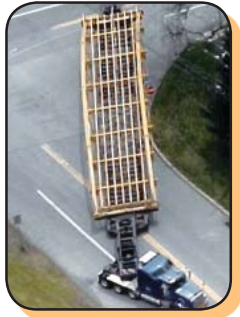
92 x 14 foot bridge was backed down Valley Road so it could be backed into the Tech Center parking lot in the proper orientation for lifting
