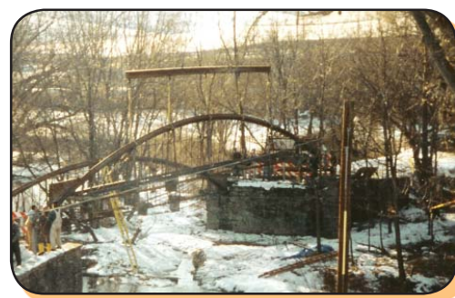
Arch No. 1 lifted from its abutments; with braces to keep the members from warping
