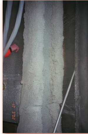
Figure 3: Structural Steel Column Protected with SFRM
