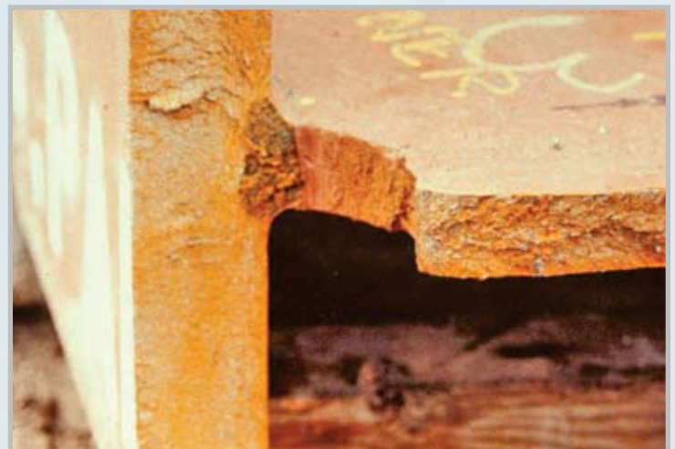
Figure 2: Brittle, low-energy fracture of a jumbo wide flange section used in the tension chord of a roof truss
