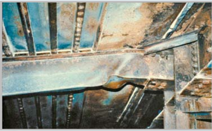
Figure 3: Local buckling of a building floor beam
