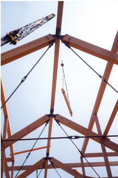
Assembled roof trusses with purlins being installed. Note three cast fittings at ridge pin.
