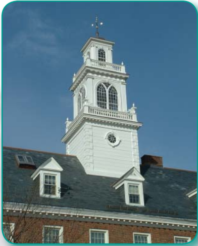
Cupola restoration included netting at balconies, ledges, and windows. Photo by Michael Teller, CBI Consulting, Inc.
