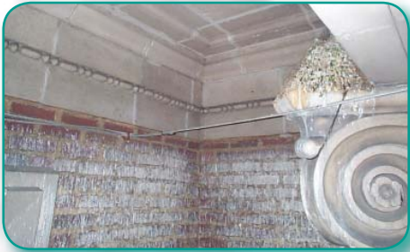
Underside of portico is protected from the weather and promotes roosting. Photo by Jim DeStefano, DeStefano Associates.
