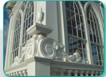
Netting virtually invisible even at close range. Photo by Michael Teller, CBI Consulting, Inc.
