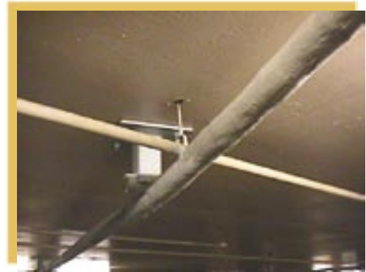
Fireproofing on external tendons
