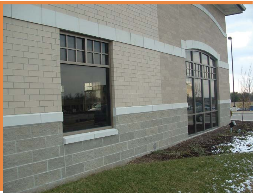
This building has a wainscot of six courses of 8 x 24-inch cast stone, 8-inch high accent bands at the top of the wainscot and near the top of the wall, and a 12-inch high accent band above the windows. A control joint was installed below the window after cracks appeared at a number of windows. It should be noted that nearly all of the head joints in the accent band over the window have hairline cracks, but they were not noticed by the Owner.
