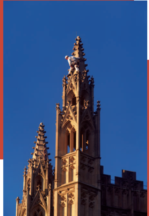
Hands-on visual inspection of stone masonry at Cleveland Tower, Princeton University, Princeton, New Jersey.
