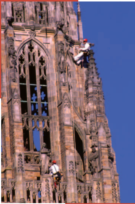
Undertaking a "stone-by-stone" conditions survey at Harkness Tower, Yale University, Hew Haven, Connecticut.
