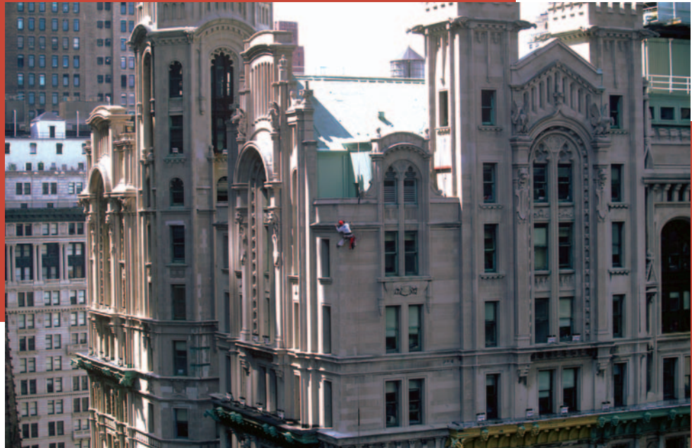
Hands-on inspection of two monumental historic structures on lower Broadway in Manhattan.
