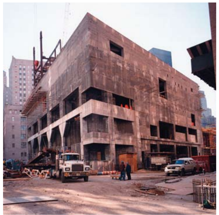
Figure 3: Robust concrete base housing Con Edison Electric substation.
