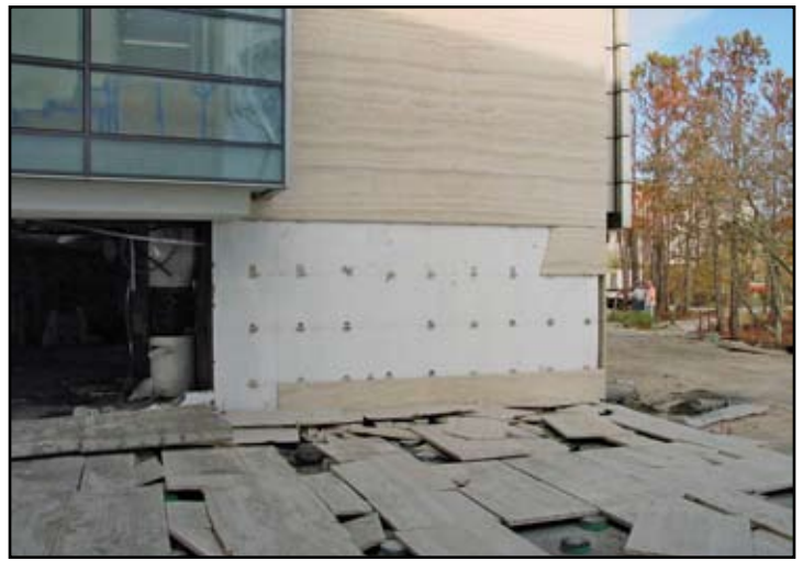
Break-Away Wall Collapse (as anticipated).
