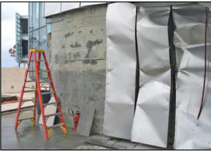
Non-Structural Cladding Damage on Core Walls.
