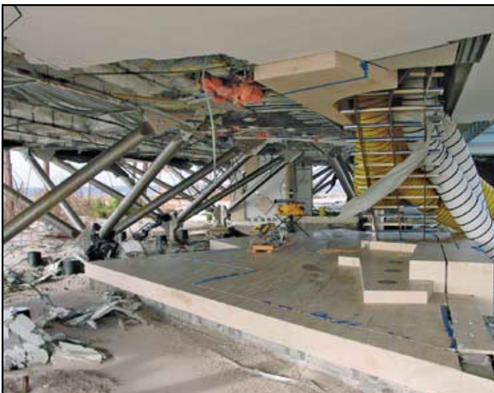
Non-Structural Damage caused by Ivan to 1 st Floor Soffit.
