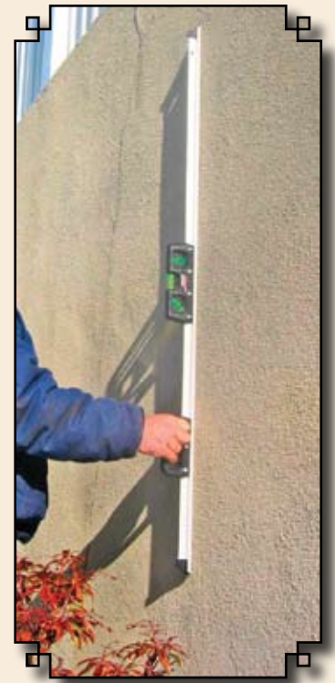
Checking verticality of a cracked retaining wall
