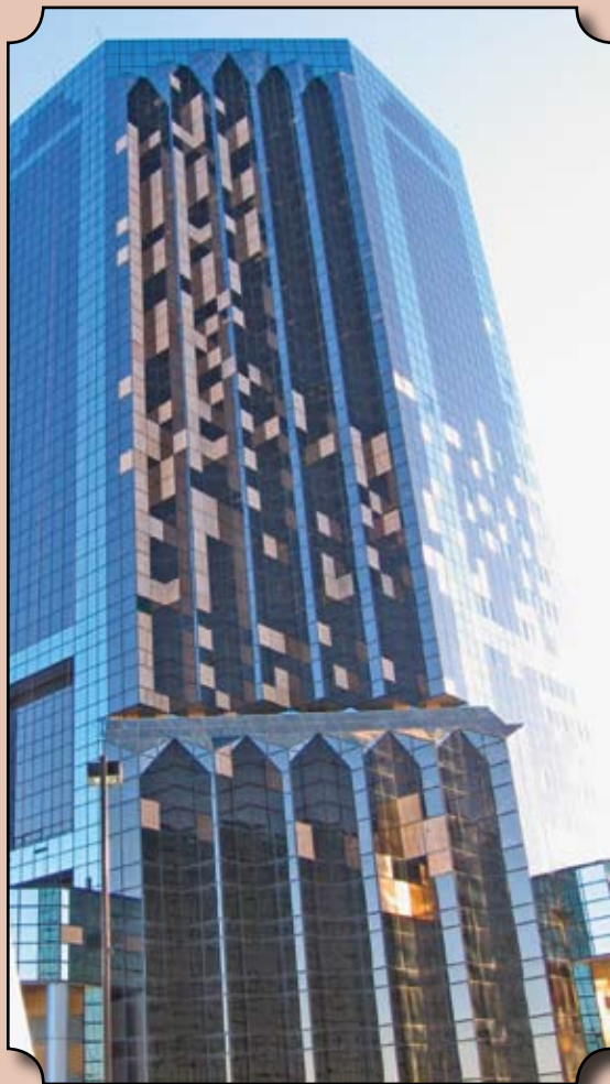
Figure 4: Curtainwall damage from Hurricane Katrina.
