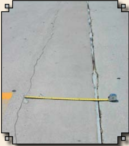
Recording a sign of distress in a precast prestressed concrete double-tee
