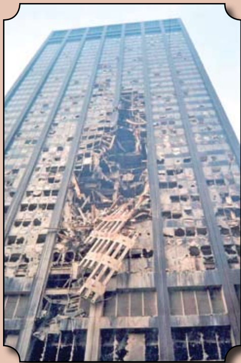
Figure 2: The loss of a column to 130 Liberty Street in New York City is an excellent example of how redundancy can prevent progressive collapse. The façade was a wind moment frame that, once a column was destroyed, acted as a vierendeel truss to span over the opening.
