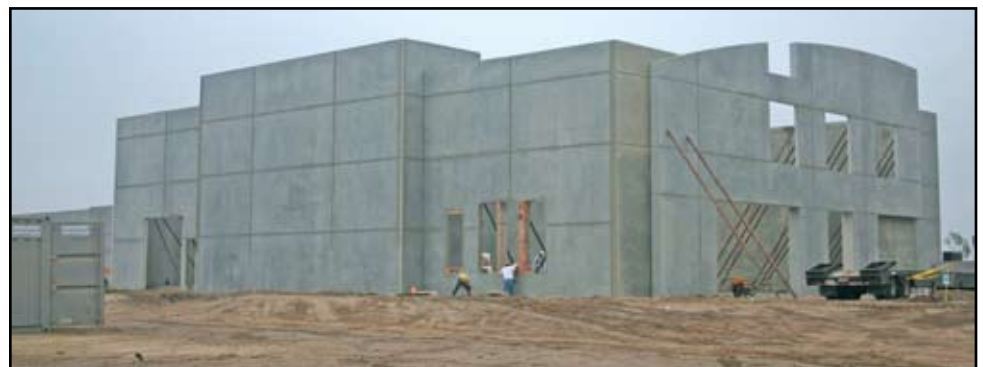
Tilt-up Building under Construction. Cottonwood Christian Center, Cypress, CA. Courtesy of R.M. Byrd Assoc., Ontario, CA.
