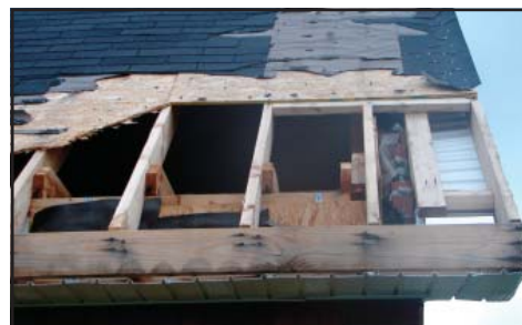
Figure 4: Roof sheathing damage at the corner of a roof, fastener spacing was in excess of the code minimum
