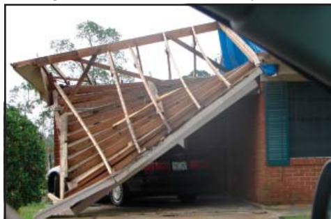
Figure 2: Carport collapsed and structure breached
