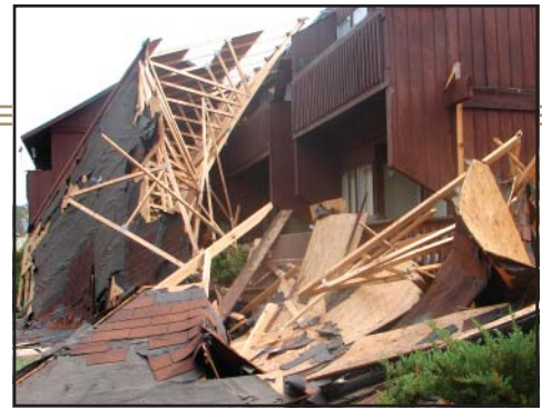
Figure 3a: Multi-family condominium roof collapse
