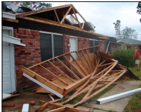
Figure 1: Porch overhang collapsed due to poor anchorage between columns (white) and foundation
