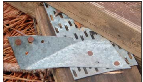
Figure 3c: Truss to top plate connected using hurricane strap but only two nails instead of four nails
