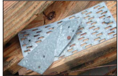
Figure 3b: Truss to top plate connected using hurricane strap but only one nail instead of four nails
