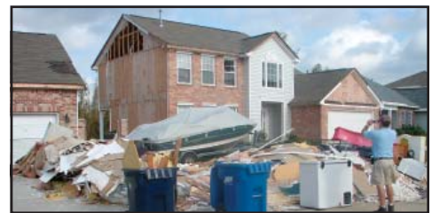
Figure 5: Non-structural, foam-substrate, insulating sheathing panels failed at the gable end
