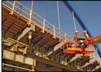
Workers stressing the hanger at the center diaphragm over the temporary bent.
