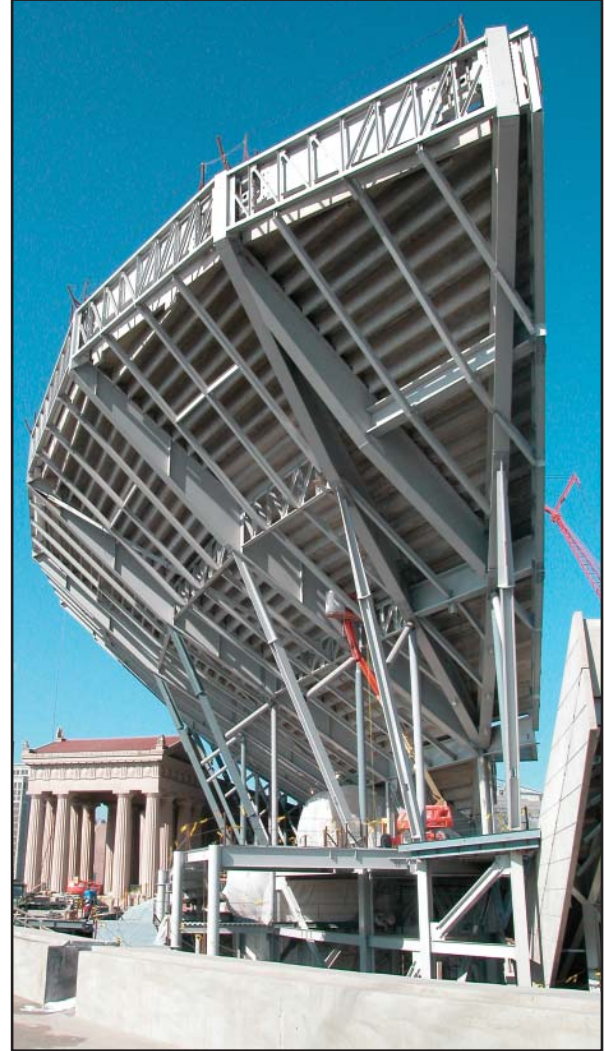
Northwest view of the underside of the West Grandstand with the tuned mass dampers (TMDs) visible at the top. Photo courtesy of Thornton-Tomasetti Group.
