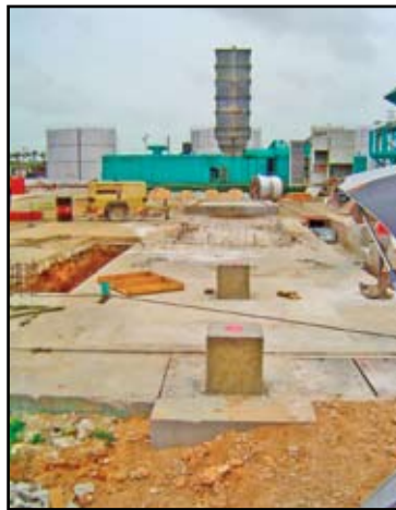
Figure 1: Foundation Site. Note staining and chipped areas to the right of the generator
