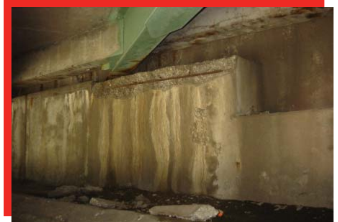
Figure 1c: Typical Corrosion problems: Abutment Wall
