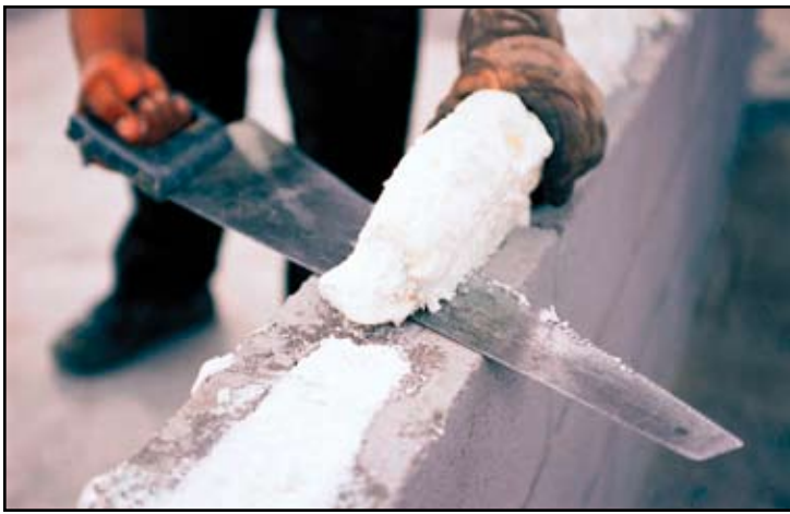
Figure 3: Polyurethane insulation is sprayed into the wall interior, allowed to expand, harden and dry. The excess is cut flush to the block.
