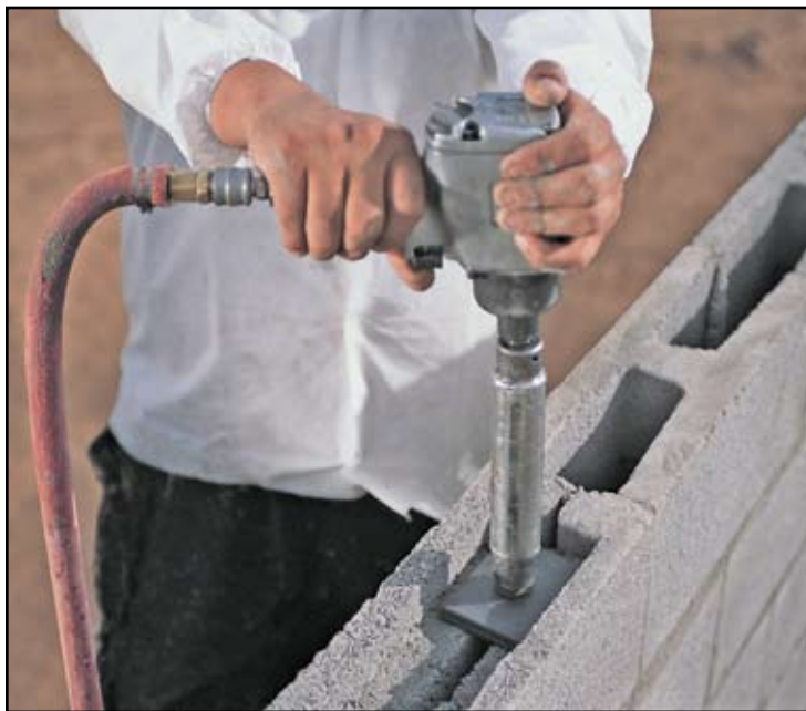
Figure 2: Once the walls are in place, the steel rods are tensioned to a pre-engineered force of 7400 pounds using impact wrenches.
