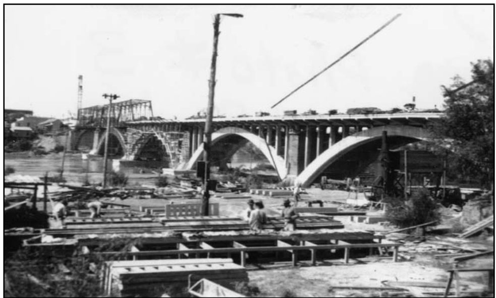
International Bridge over the Rio Grande River, Laredo, Texas, 1921. The 1,600-foot long, multi-span, concrete arch structure was the longest and first-of-its-kind in the area. (Photo courtesy of H. Douglas Steadman)
