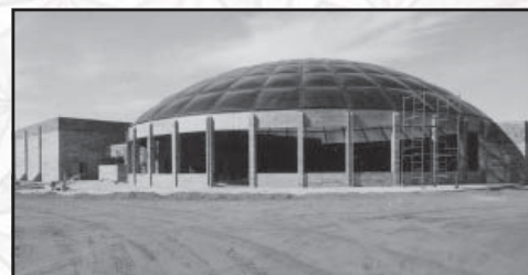
Geodesic dome with plastic panel roofing for the City Recreation and Pool Building, North Platte, Nebraska. Photo courtesy of Richard Weingardt Consultants, Inc.
