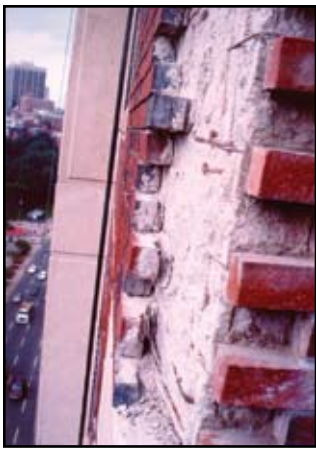
Figure 4: Panel with brick removed showing reinforcement in the concrete and the ragged freeze thaw fracture at veneerface
