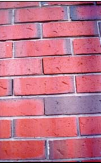
Figure 1: Raked mortar joints at brick veneer
