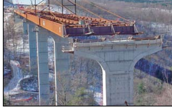
Launching of the Clifford Hollow Bridge, Hardy, West Virginia. Courtesy of HDR Engineering, Inc.
