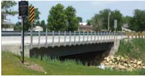
New Jesup South Bridge designed with standardized steel beams with eSPAN140 tool.
