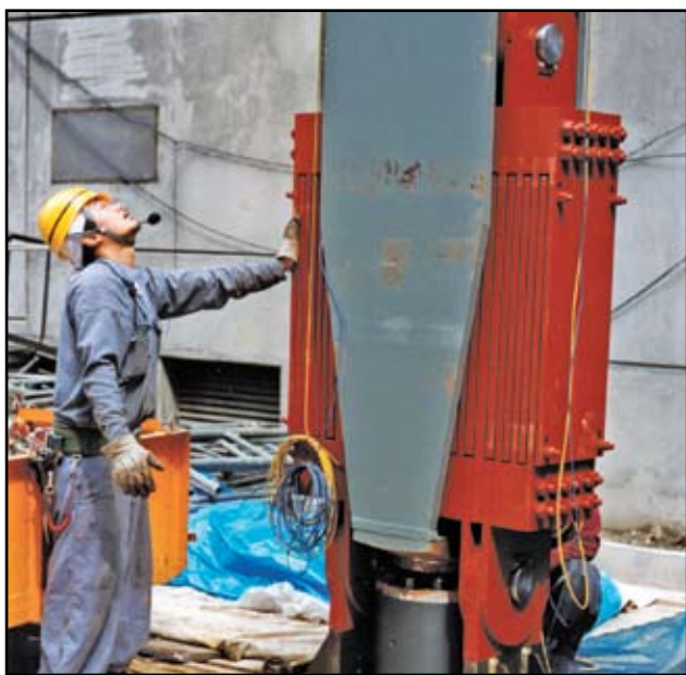
A visco-elastic damper provides for a “stepping column” base connection in the Maison Hermes Building in Tokyo, Japan. ©Arup/Frank la Riviere
