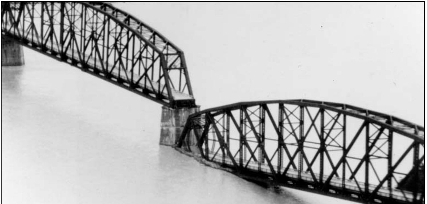
Alaska Earthquake March 27, 1964. Million Dollar Bridge on the Copper River Highway; no. 4 span off no. 4 pier. View is southwest. Courtesy of http://libraryphoto.cr.usgs.gov .
