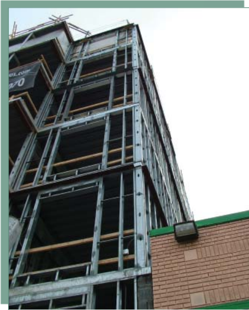
Multi-story loadbearing projects have become very popular recently, with new developments in steel-framing construction.
