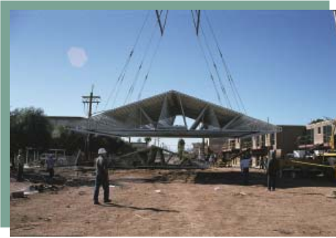
A pre-fabricated truss assembly made from cold-formed steel being “flown” into place at Davis Mothan Air Force Base. Note the rough plumbing and ductwork is already installed in the roof systems.
