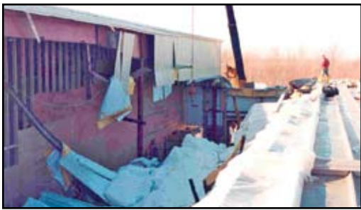
Figure 3: Overview of "link" bay section intended to support drifted snow at the junction of high- and low-roof building areas.
