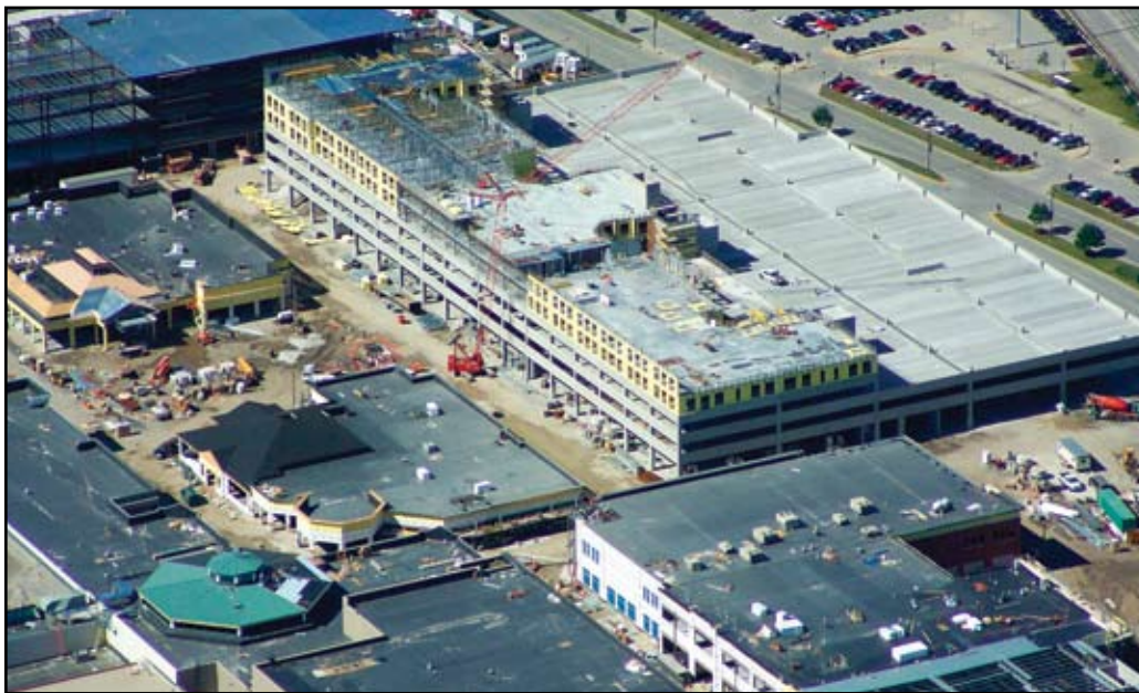
Bayshore Town Center North Parking Structure – Erection of parking and residential levels of structure.
