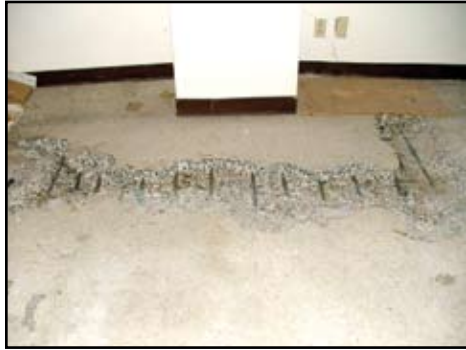
Figure 2c: Punching shear failure (Column B6 at the 3 rd floor level).
