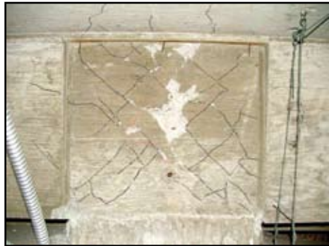
Figure 2d: Shear crack on beam-column joint (Column A4 at the 3 rd floor level).
