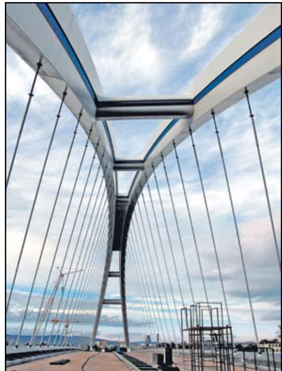
Figure 6: Apollo Bridge, Slovakian Republic - looking upward at basket handle arch and bare orthotropic steel deck prior to floating across the river. Photo courtesy of DYWIDAG Systems International, Germany.
