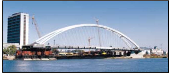
Figure 5: Apollo Bridge, Slovakian Republic. The left end of the bridge was slid on a curved steel beam onto falsework platform on top of a pontoon. Photo courtesy of DYWIDAG Systems International, Germany.
