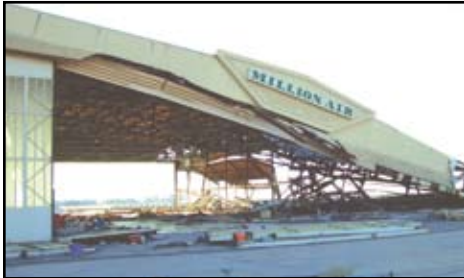
Partial Collapse of the Million Air Hanger, Lakefront Airport, New Orleans, LA., Courtesy of Ed Huston, Smith & Huston, Inc., All Rights Reserved.
