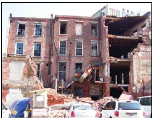
Partial Collapse of the building at 109 Tchoupitoulas, New Orleans, LA., Courtesy of Ed Huston, Smith & Huston, Inc., All Rights Reserved.
