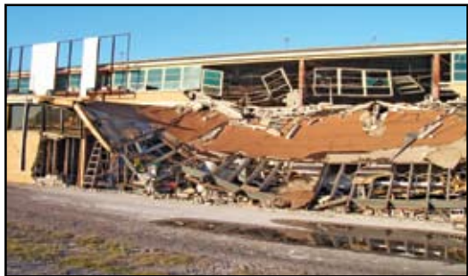
Partial Collapse of the Wendell Hanger, Lakefront Airport, New Orleans, LA., Courtesy of Ed Huston, Smith & Huston, Inc., All Rights Reserved.
