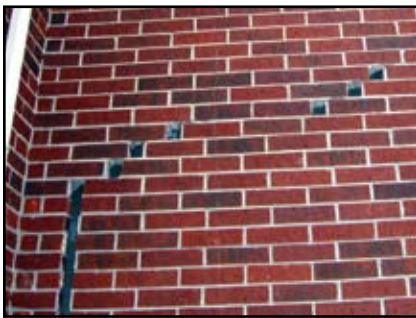
Figure 1: The major crack in the corner of the south wing brick wall.
