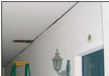
Figure 3: Gap between the ceiling and the siding wall on the 3 rd floor.
