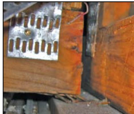
Figure 4: Bearing of the wood roof truss. Note the pulled-out nails.
