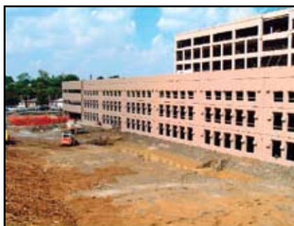
Exterior shear wall panels. “Columns” in panels are at six feet on center and projecting brackets are designed to support double-tee stems of future addition.
