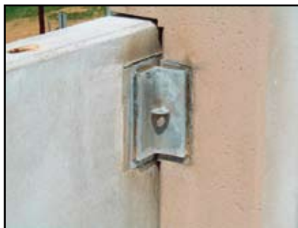
Angle welded to top of spandrel beam and column transfers tension from negative moment at joint. (Ring was used to suspend angle when dipped in galvanizing tank).
