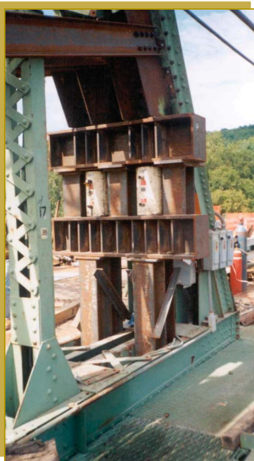
Auxiliary truss member, transfer beam, and jacks for structural lifting operations of Dam 6 at Lock E10 on the Erie Canal; Town of Florida, NY
