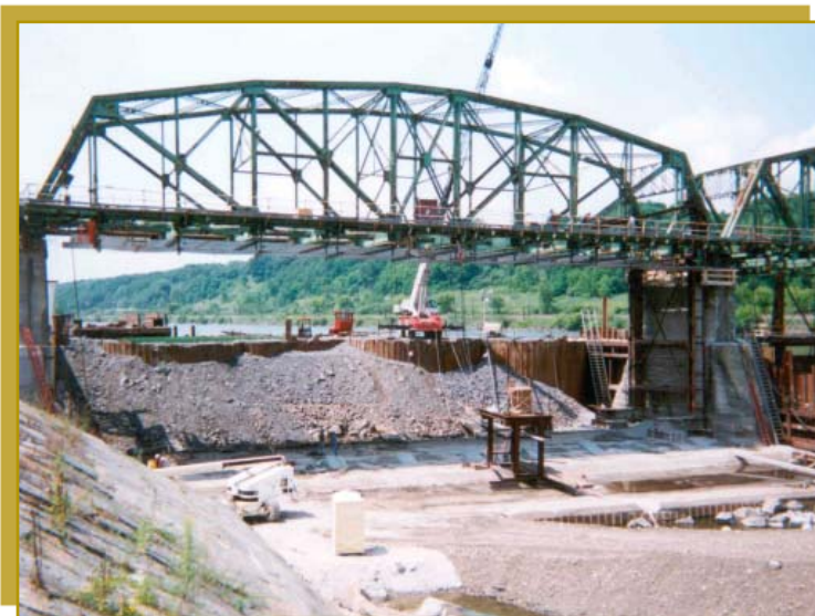
Global photo of structural lifting operations of Dam 6 at Lock E10 on the Erie Canal; Town of Florida, NY
