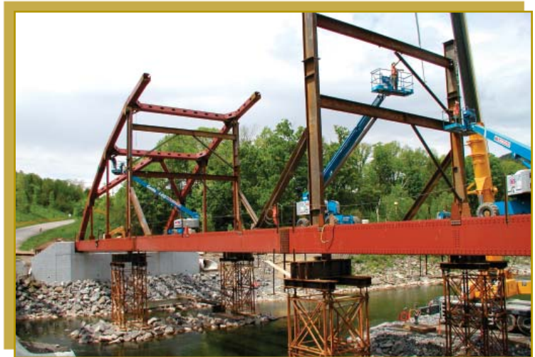
Erection of tied-arch bridge in Schoharie, NY. Photo courtesy of D.A. Collins Construction Company, Inc.
