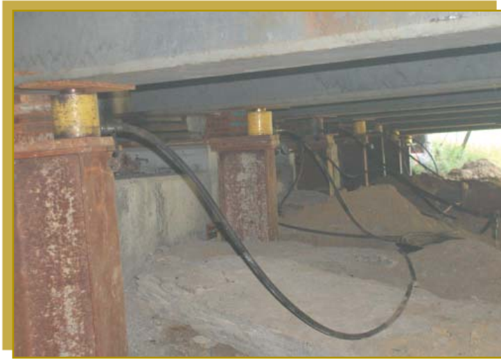
Structural lifting of multi-girder bridge at the abutment; Cobleskill, NY. Photo courtesy of D.A. Collins Construction Company, Inc.
