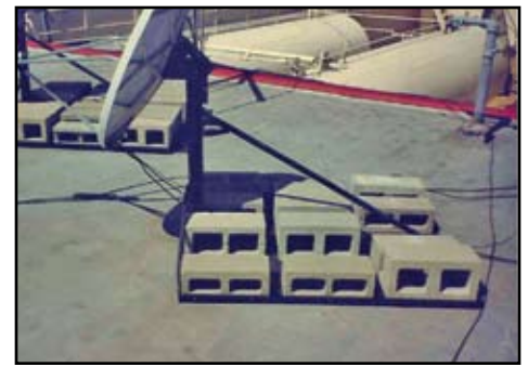
Figure 4: Unanchored Roof Antenna Base Anchorage.
