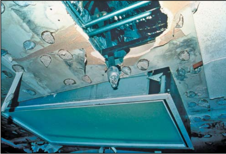
Figure 6: Broken Fire Sprinkler Pipe and Water Damage. Photo by Bob Reitherman, courtesy of EERI.
